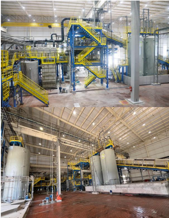
Battery Breaker Machine
